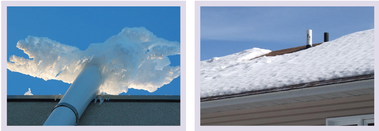
Figure 15 - Examples of a sub-slab depressurisation system external roof exhaust stack in a cold weather region with one case of ice build-up at the top (Photo courtesy CMHC)
