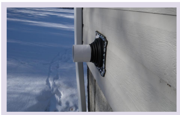
Picture #- Example of a ground level exhaust discharge
