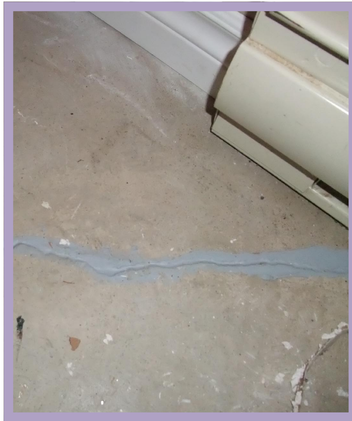
Picture 9 – Example of a sealed crack on the concrete slab
