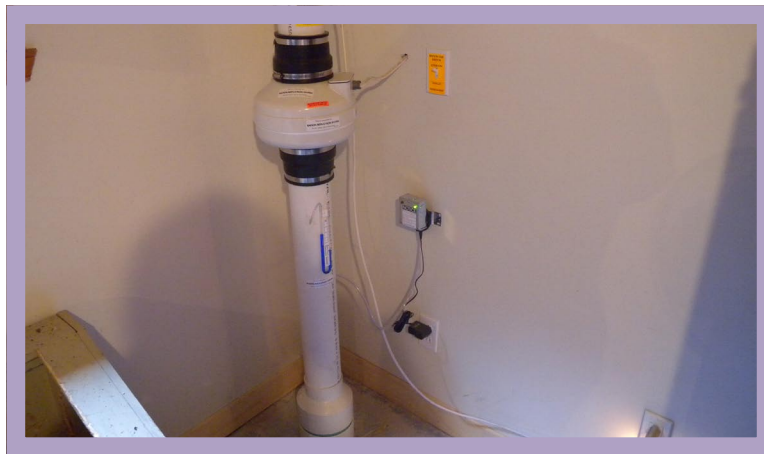
Picture 4 – Fan installed in the basement
