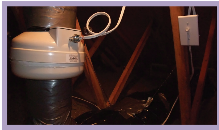
Picture 3 – Fan installed in the attic
