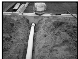
• Pipe laid in subgrade with approximately 1-inch of fill above. • Pass loop through intermediate footings
