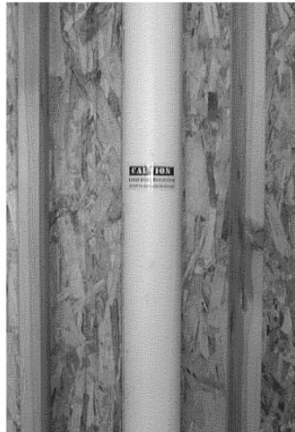
Label all portions of visible pipe "Radon Reduction System"
